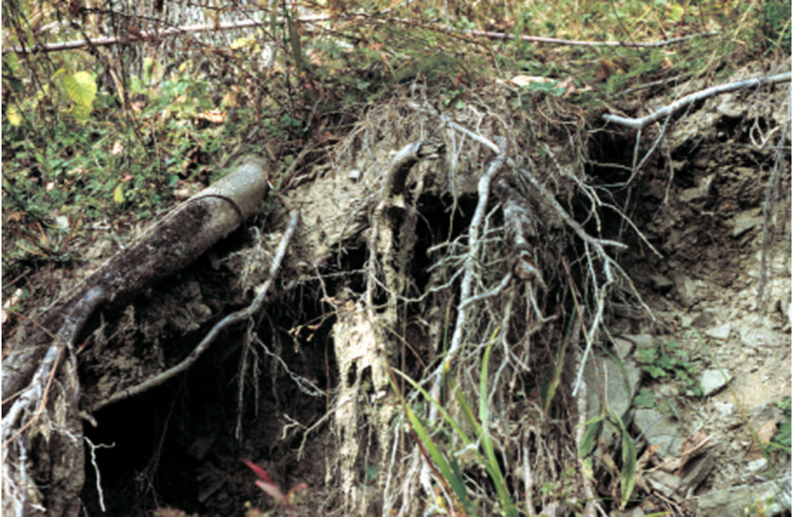
Photograph 16. Example of tree root damage resulting from subsidence at Lee property
