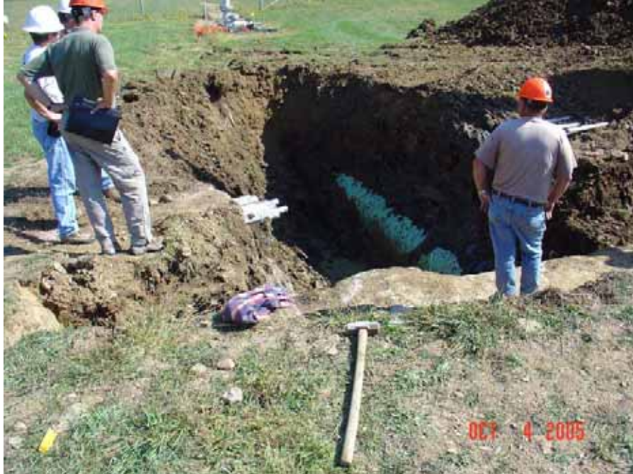
Photo IV-13e: DEP Photograph taken on October 4, 2005 showing a Texas Eastern pipeline being exposed for repairs.
