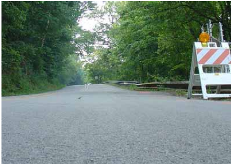
Photo II-34 : DEP photograph, taken August 11, 2005, shows the heaving of Bristoria Road.
