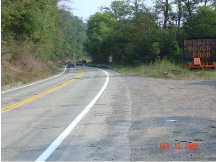
Photo IV-6a: DEP Photograph taken on September 15, 2005 showing milled and patched road bump in eastbound lane of Route 21.
