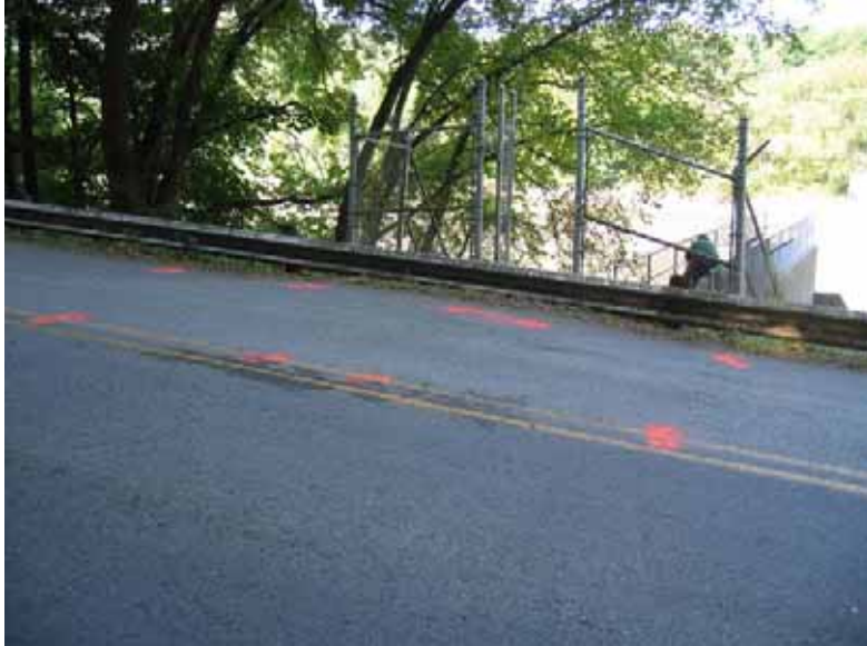
Photo II-35 : DEP photograph, taken August 16, 2005, shows the heaving of Bristoria Road.
