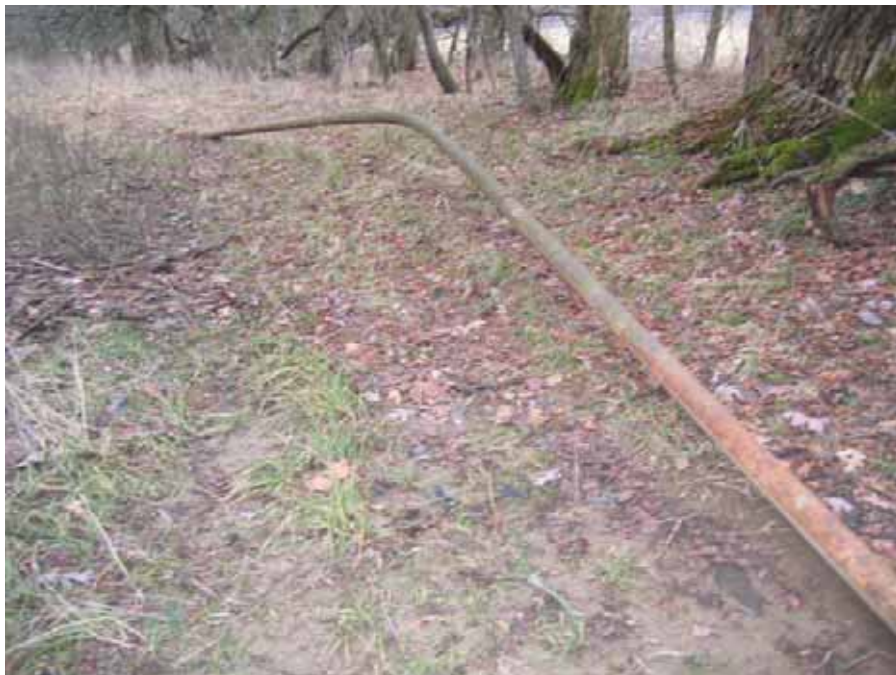
Photo IV-14d: DEP Photograph taken on February 7, 2008 showing pipeline heave.
