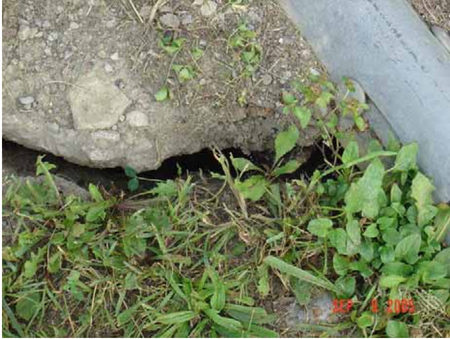
Photo IV-5e: DEP Photograph taken on September 9, 2005 showing close-up of ground separation at northeastern guide rail mooring of Lazear Lane Bridge.
