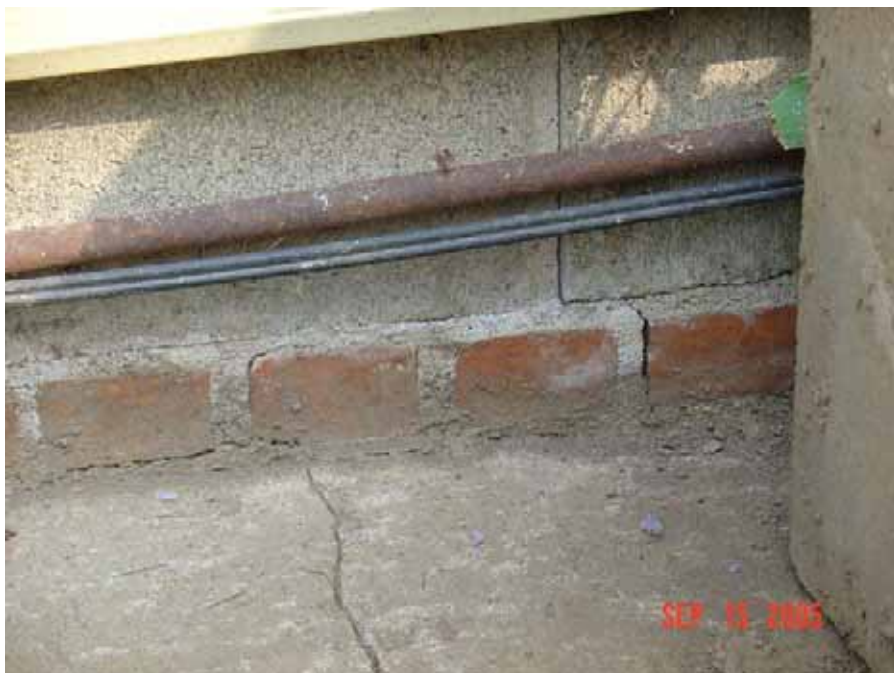
Photo IV-9b: DEP Photograph taken on September 15, 2005 showing close-up of minor cracks in Bottinelli Residence.
