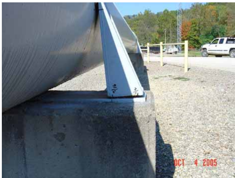
Photo IV-13d: DEP Photograph taken on October 4, 2005 showing movement of a Texas Eastern pipeline.
