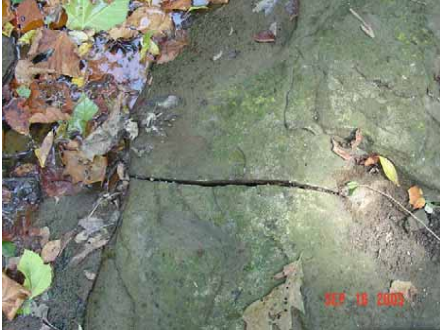
Photo IV-11e: DEP Photograph taken September 16, 2005 showing crack in bedrock within streambed.
