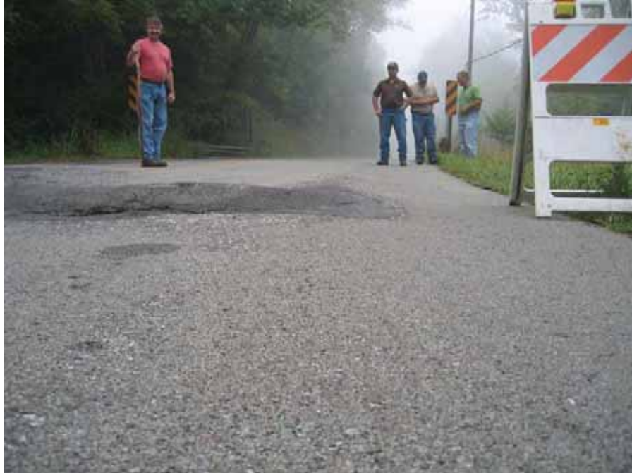
Photo IV-1a: DEP Photograph taken August 15, 2005 showing road bumps within southbound lane of Bristoria Road.
