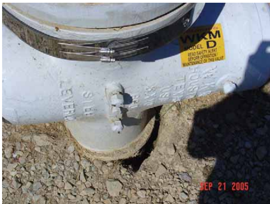
Photo IV-13c: DEP Photograph taken on September 21, 2005 showing ground movement around a Texas Eastern pipeline.
