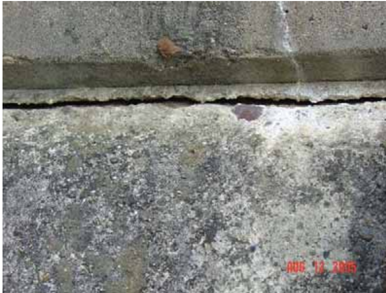
Photo II-29 : DEP photograph, taken August 12, 2005, shows a separation in the horizontal construction joint on the right (east) side of the dam.
