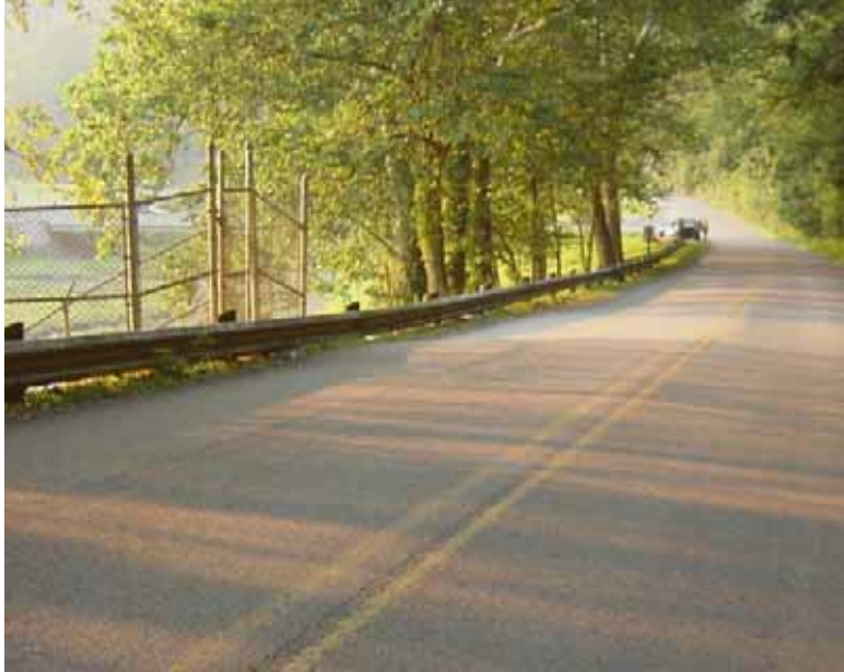
Photo II-33 : DEP photograph, taken July 30, 2005, shows another view of the buckling of Bristoria Road.
