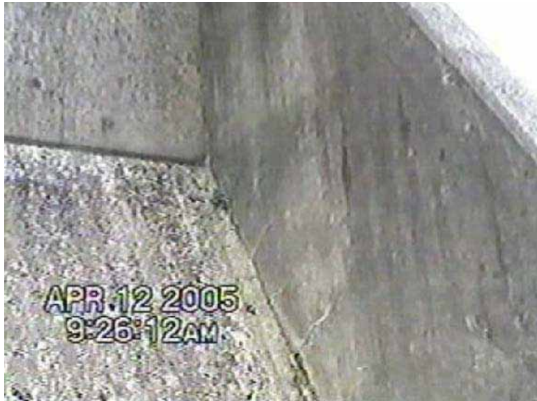
Photo II-36 : CPCC video taken April 12, 2005 shows little to no cracking in this area at the time of the video.
