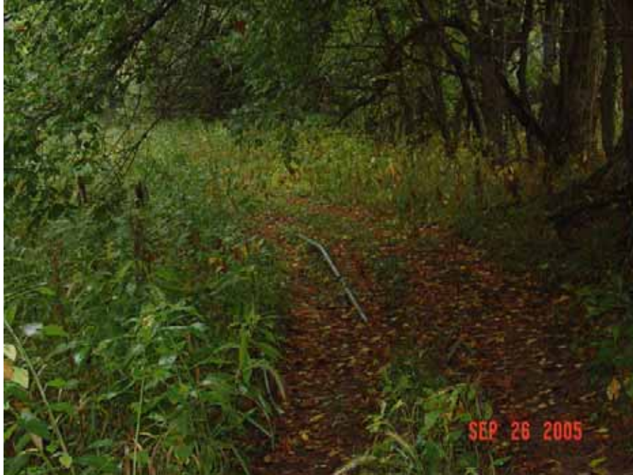
Photo IV-14a: DEP Photograph taken on September 26, 2005 showing pipeline heave upon discovery by the DEP.
