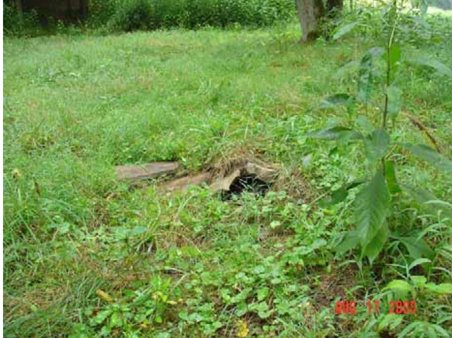
Photo IV-4a: DEP Photograph taken on August 17, 2005 showing ground heave.
