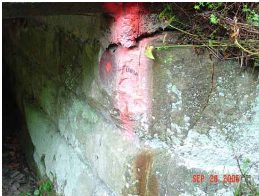
Photo IV-2d: DEP Photograph taken on September 26, 2005 showing movement within southeast corner of Bristoria Road Bridge.
