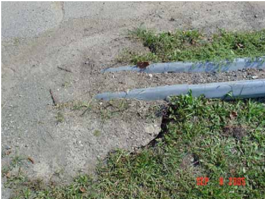
Photo IV-5d: DEP Photograph taken on September 8, 2005 showing ground separation at northeastern guide rail mooring of Lazear Lane Bridge.
