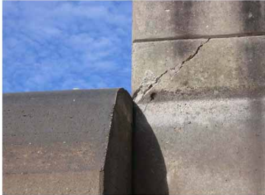
Photo 3. Sheared Concrete where Right Non-Overflow meets Spillway (Photo December 2006)
