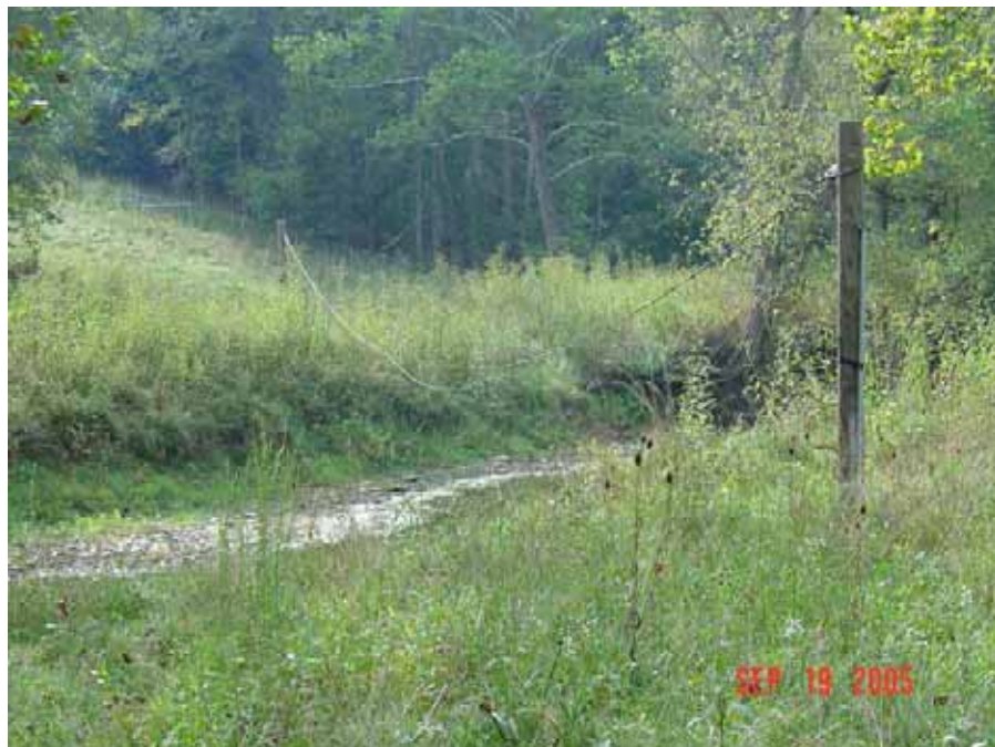
Photo IV-12f: DEP Photograph taken on September 19 2005 showing sag in pipeline marker cable crossing streambed.
