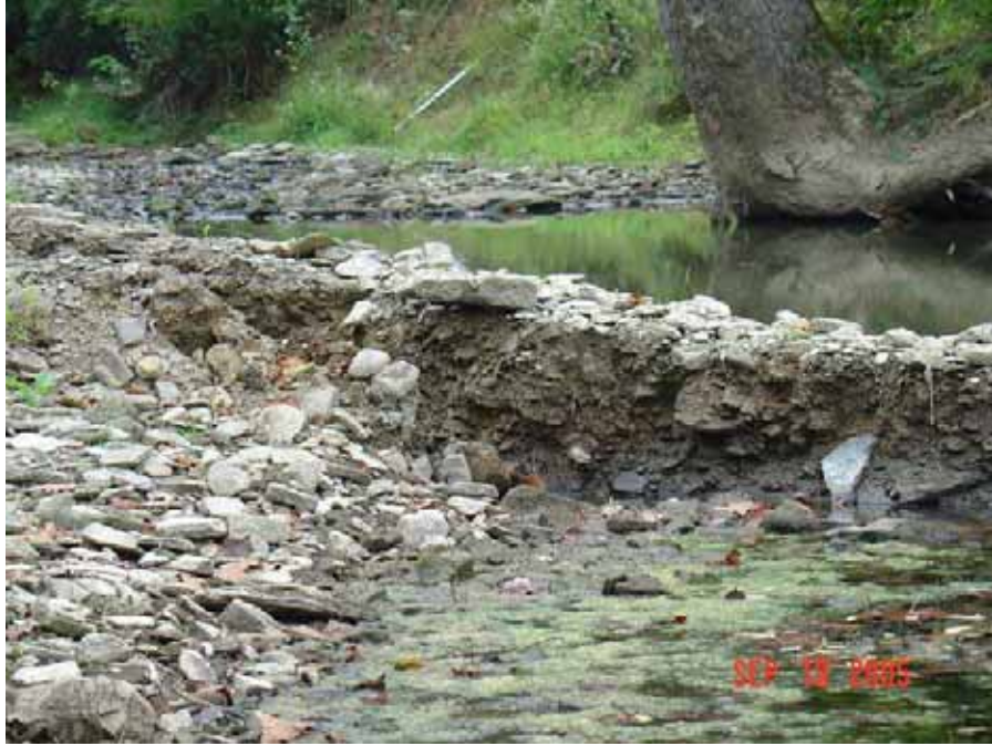
Photo IV-12c: DEP Photograph taken on September 19 2005 showing close-up of Texas Eastern pipeline heave looking upstream.
