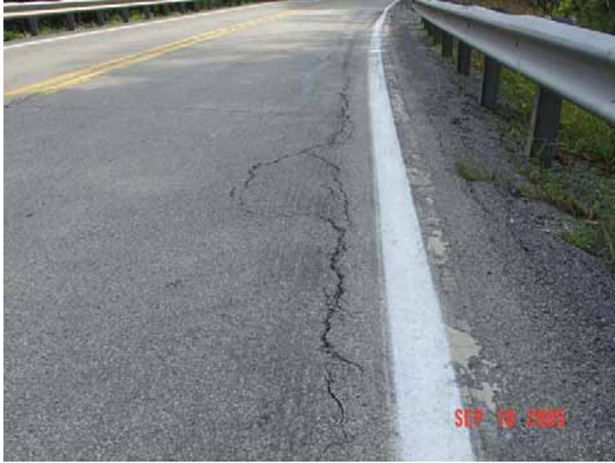
Photo IV-8a: DEP Photograph taken on September 19, 2005 showing cracks within westbound lane of Route 21.
