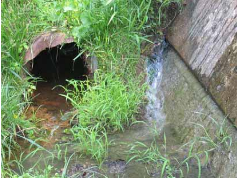
Photo II-26 : DEP photograph, taken July 20, 2005, shows the seepage in this area has increased.
