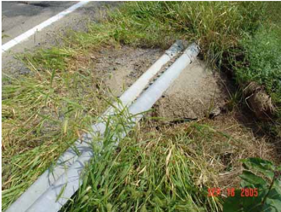
Photo IV-10b: DEP Photograph taken on September 16, 2005 showing ground separation around southeastern guide rail mooring.
