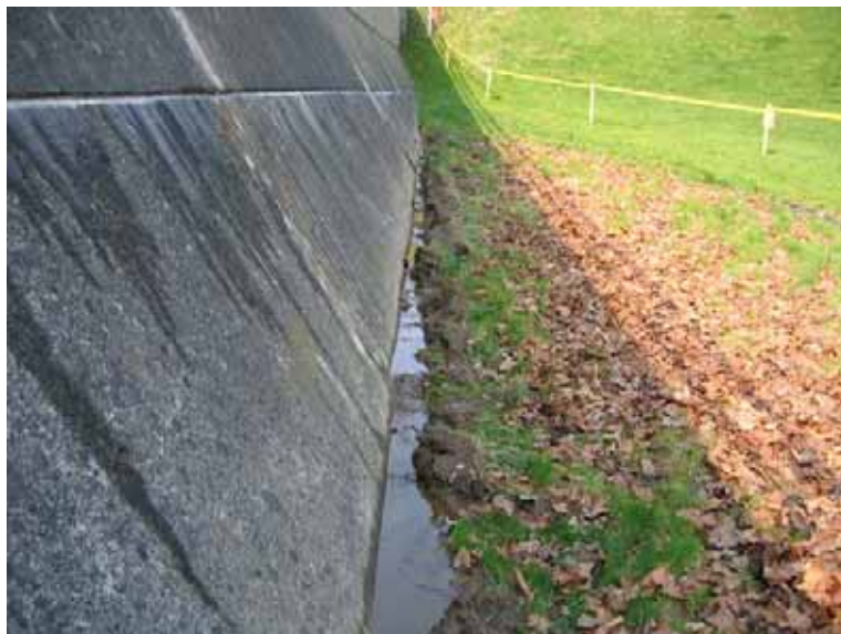
Photo II-12 : DEP photograph, taken April 18, 2005, shows the seepage in this area.
