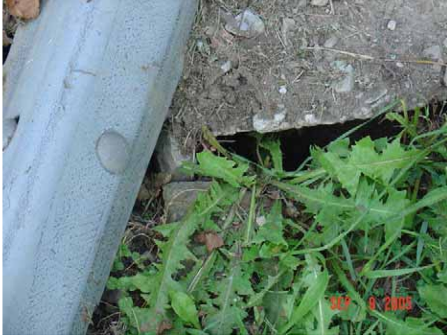
Photo IV-5c: DEP Photograph taken on September 9, 2005 showing close-up of ground separation at southeastern guide rail mooring of Lazear Lane Bridge.
