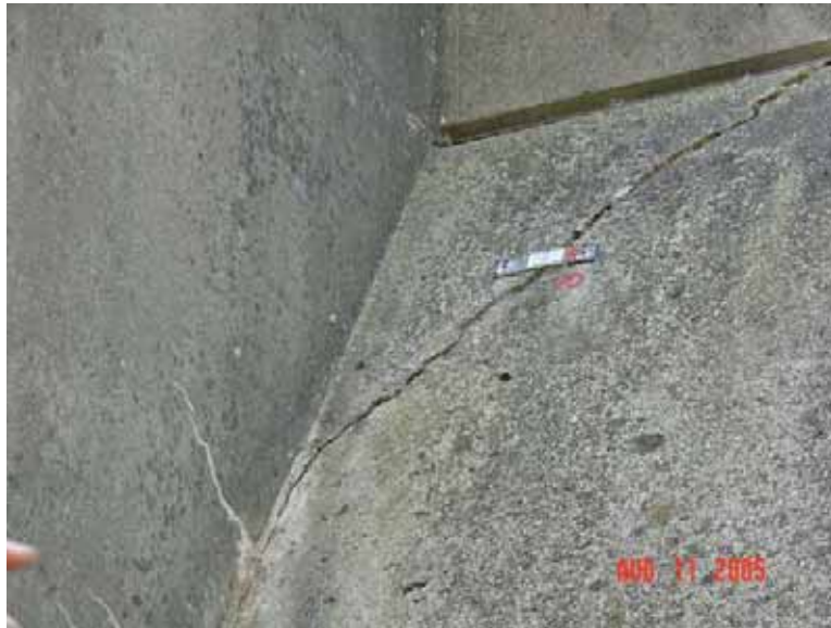
Photo II-18 : DEP photograph, taken August 11, 2005, shows the cracking in this area has become more severe.
