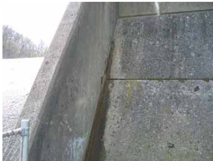
Photo II-17 : DEP photograph, taken April 18, 2005, shows minimal cracking in this area
