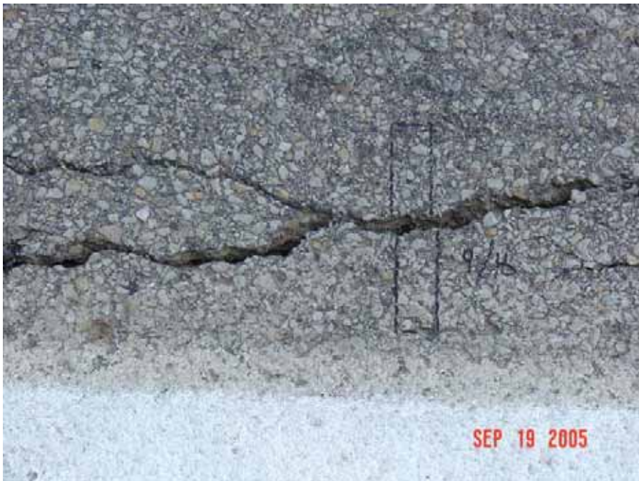
Photo IV-8b: DEP Photograph taken on September 19, 2005 showing close-up of cracks and movement in westbound lane of Route 21.
