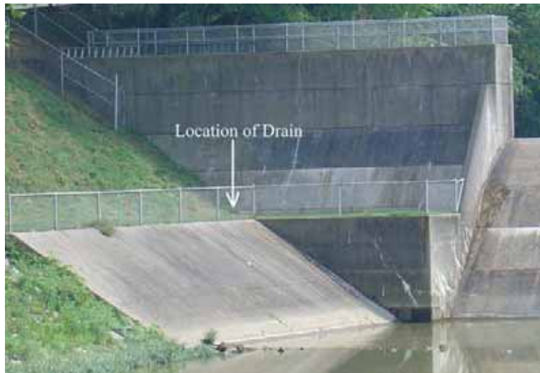
Photo II-24 : Photograph showing the location of the drain referenced above.
