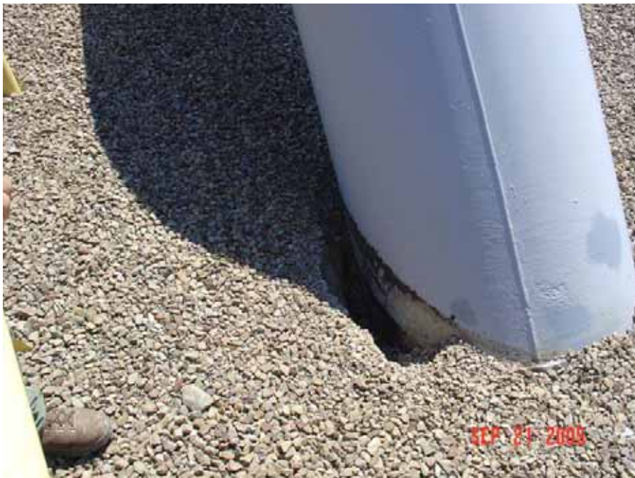
Photo IV-13b: DEP Photograph taken on September 21, 2005 showing ground movement around Texas Eastern pipeline.
