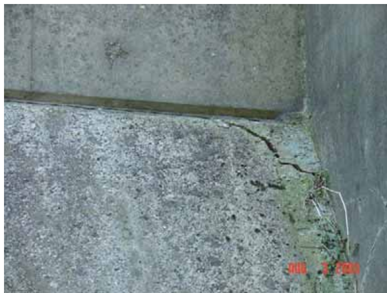
Photo II-37 : DEP photograph taken August 3, 2005 shows the damage in this area has become much more severe.
