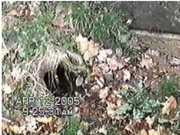
Photo II-25 : CPCC video, taken April 12, 2005, shows there is little to no drainage coming from the drain or the area around the drain.
