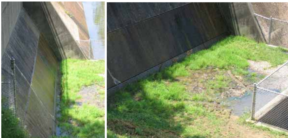
Photo II-22 and II-23 : DEP photograph, taken July 20, 2005, shows a large amount of water pooling in the area near the base of the dam.
