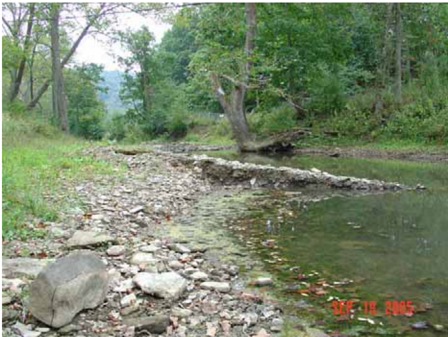
Photo IV-12b: DEP Photograph taken on September 19 2005 Texas Eastern pipeline heave looking upstream.
