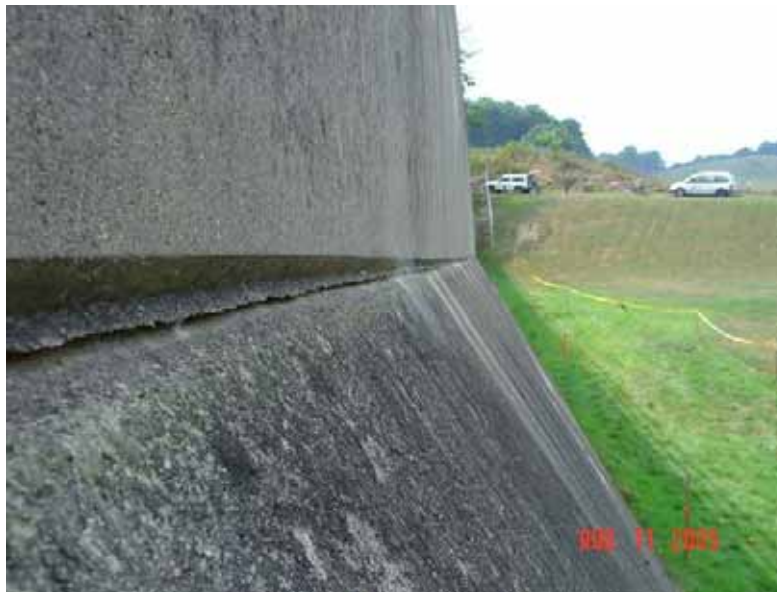
Photo II-19 : DEP photograph, taken August 11, 2005, shows separation of the second horizontal joint from the crest of the dam.
