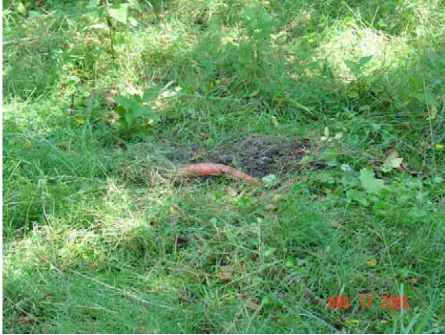
Photo IV-3a: DEP Photograph taken on August 17, 2005 showing gas line beginning to heave out of ground.
