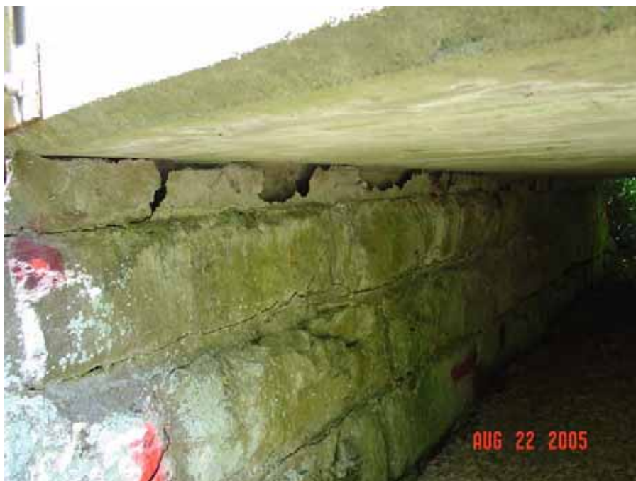
Photo IV-2b: DEP Photograph taken on August 22, 2005 showing movement of the western end of Bristoria Road Bridge.
