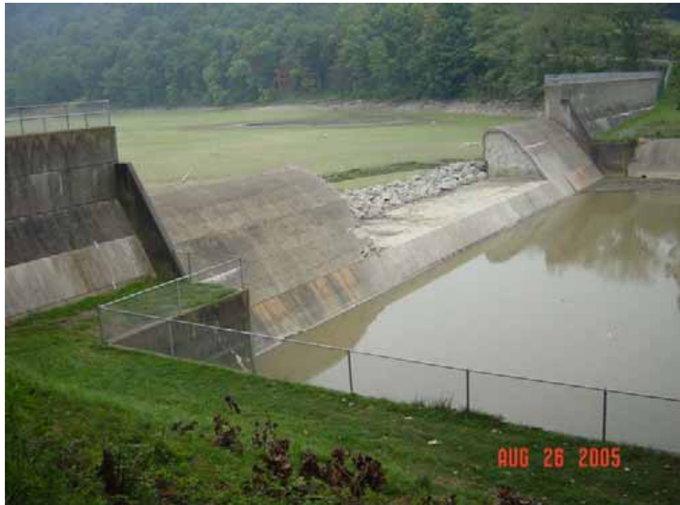
Photo II-9: DEP photograph, taken August 26, 2005, shows the dam breached.
