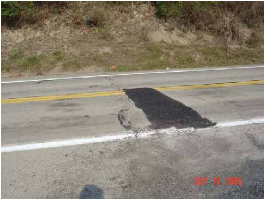
Photo IV-6b: DEP Photograph taken on September 15, 2005 showing side view of milled and patched road bump in eastbound lane of Route 21.
