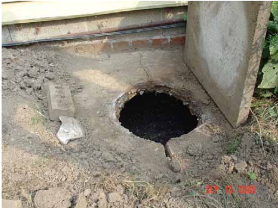
Photo IV-9a: DEP Photograph taken on September 15, 2005 showing minor cracks in Bottinelli Residence.
