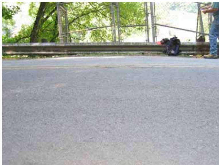
Photos II-32 : DEP photograph, taken August 1, 2005, shows the buckling of Bristoria Road. Note the distance from the road to the bottom of the guard rail is much less in this area.
