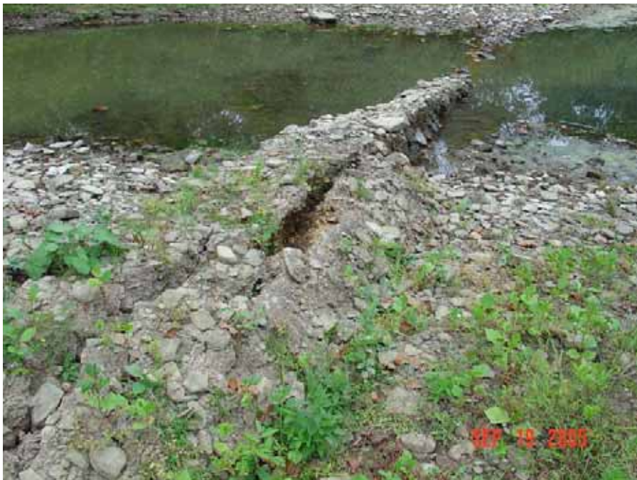
Photo IV-12d: DEP Photograph taken on September 19 2005 showing Texas Eastern pipeline heave crossing streambed.
