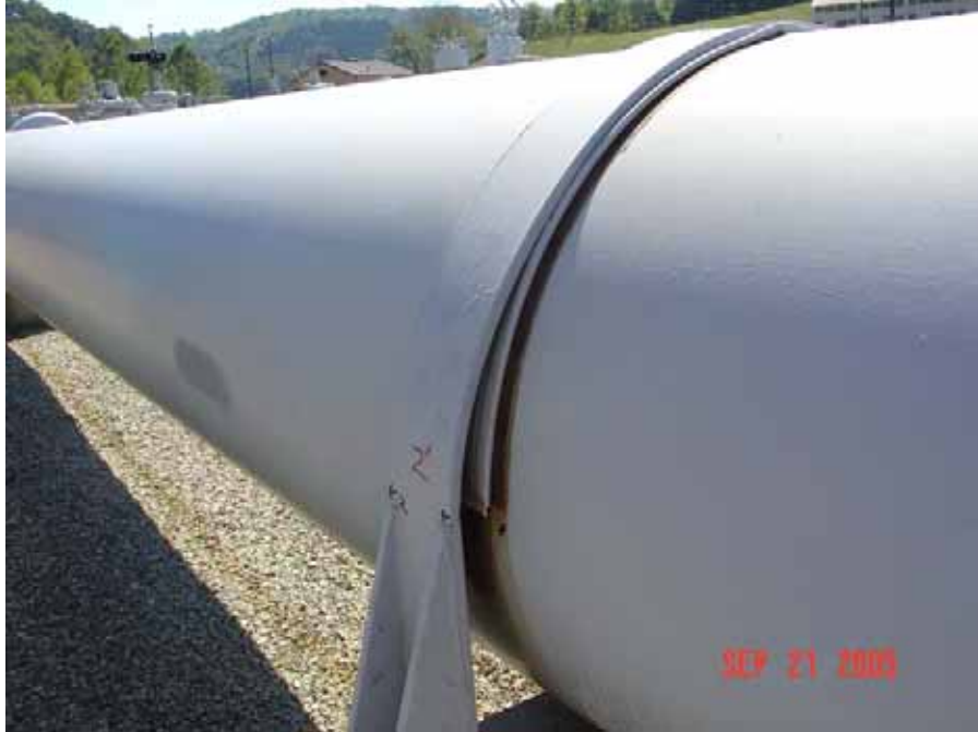
Photo IV-13a: DEP Photograph taken on September 21, 2005 showing movement of a Texas Eastern pipeline.
