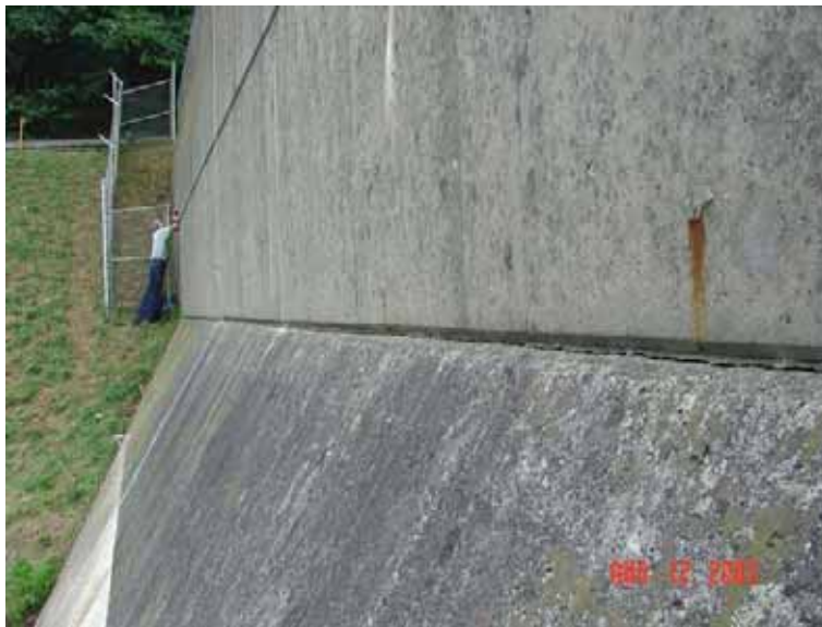
Photo II-30 : DEP photograph, taken August 12, 2005, shows a separation in the horizontal construction joint on the right (east) side of the dam.
