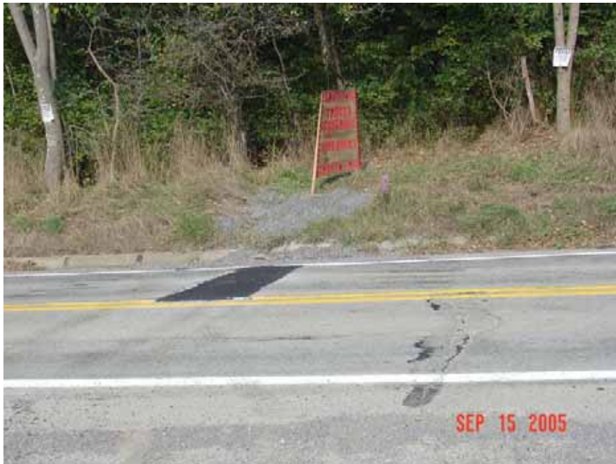
Photo IV-7b: DEP Photograph taken on September 15, 2005 showing side view of milled and patched road bump in westbound lane of Route 21.
