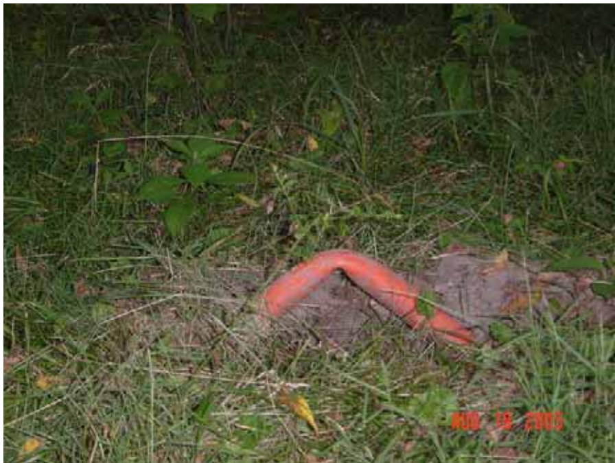
Photo IV- 3b: DEP Photograph taken on August 19, 2005 showing gas line heave 2 days after it was discovered by DEP.
