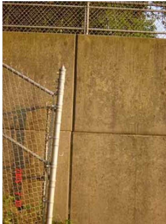
Photo II-28 : DEP photograph, taken July 30, 2005, shows the vertical and horizontal joints no longer line up in this area.
