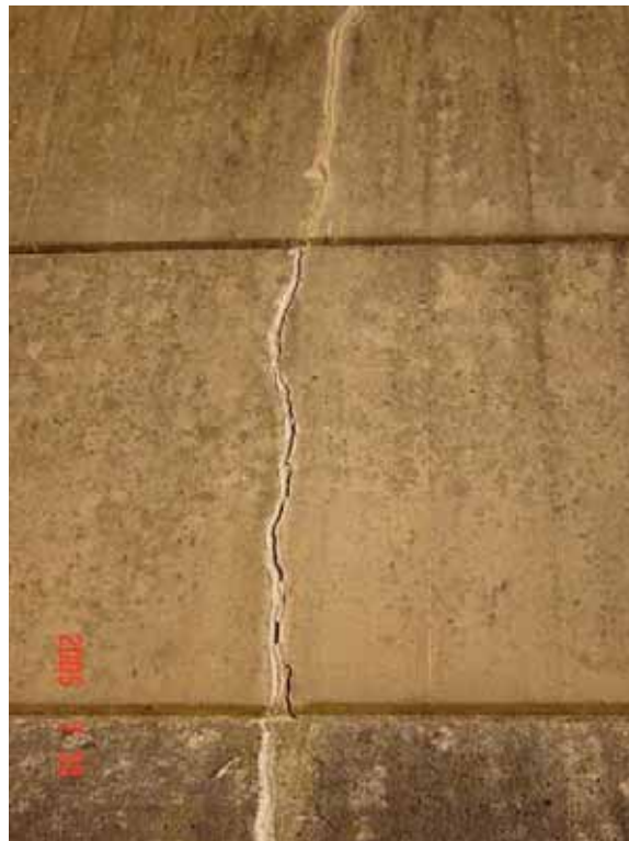
Photo II-14 : DEP photograph, taken July 30, 2005, shows the damage to this area has become more severe.
