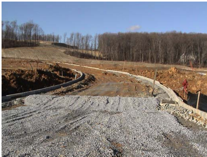
Figure 5.7-2 Example of site development with extreme soil compaction on steep slope
