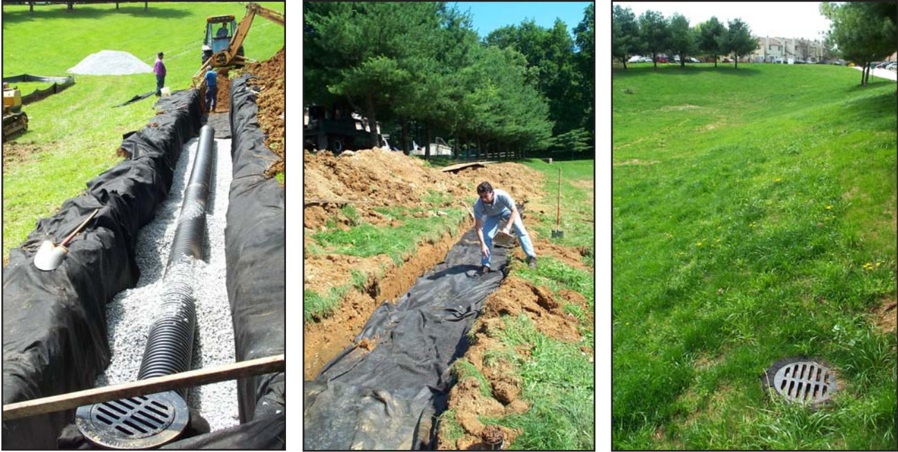
Figure 6.4-6. (From left to right) Installation of Inlets and Control Structure; Non-woven Geotextile is folded over Infiltration Trench; Stabilized Site
