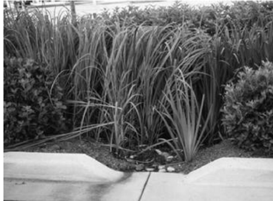
Figure 6.5-3. Curb cut inlet for a rain garden in a parking island (PGDER, 2002)
