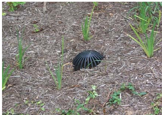
Figure 6.5-5. Domed riser provides positive overflow during extreme storm events
