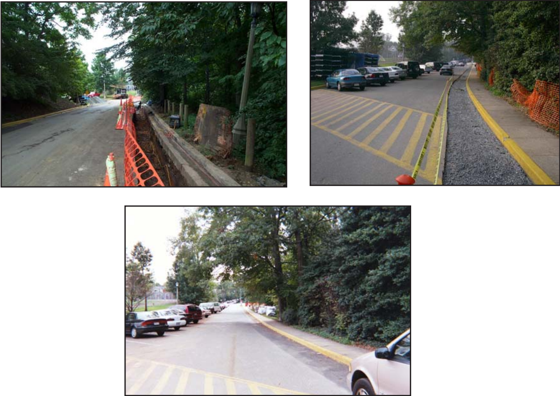
Figure 6.4-7. (Clockwise from top left) Infiltration Trench is on downhill side of roadway; Infiltration Trench is Installed; Infiltration Trench is paved with standard pavement material
