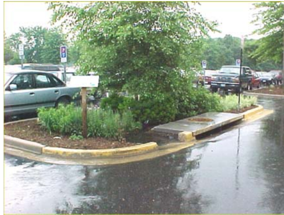
Figure 6.5-14. Parking lot island with recharge bed (LIDC)
