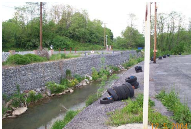
Figure 7-7. Gabion boxes encroach on the riparian section and constrain the natural floodplain.
