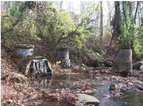
Figure 7-9. Combined Sewer Overflow to the Darby Creek in Philadelphia.
