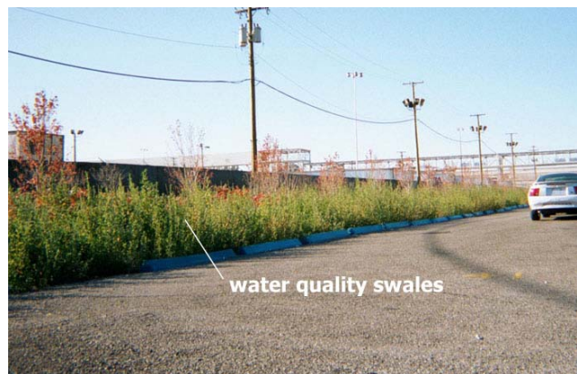
Figure 7-19. Porous pavement vehicle staging lot with adjacent water quality swale.
