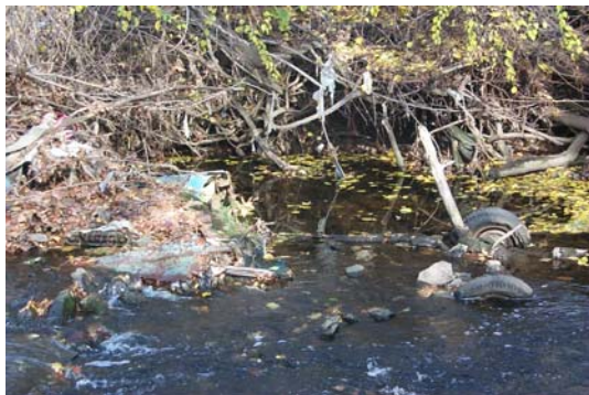
Figure 7-11. Trash and debris accumulate in urban streams.
