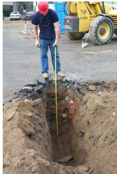
Figure 7-5. Urban soils, as found in West Philadelphia above, are generally compacted and disturbed
