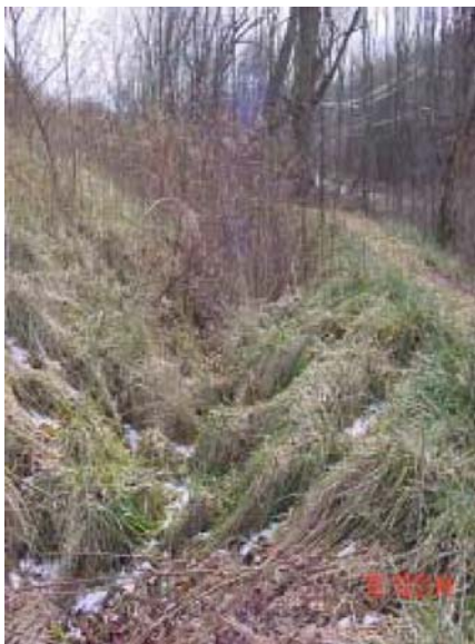
Figure 34. Narrow, vegetated infiltration trenches/berms follow land contours and take on a naturalized appearance.
