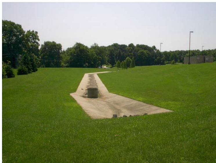
Figure 10-25 Existing sinkhole-plagued detention basin
