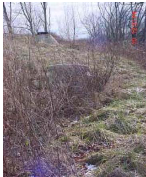
Figure 35. This trench/berm has a subsurface energy dissipater to reduce the velocity of entering stormwater.
