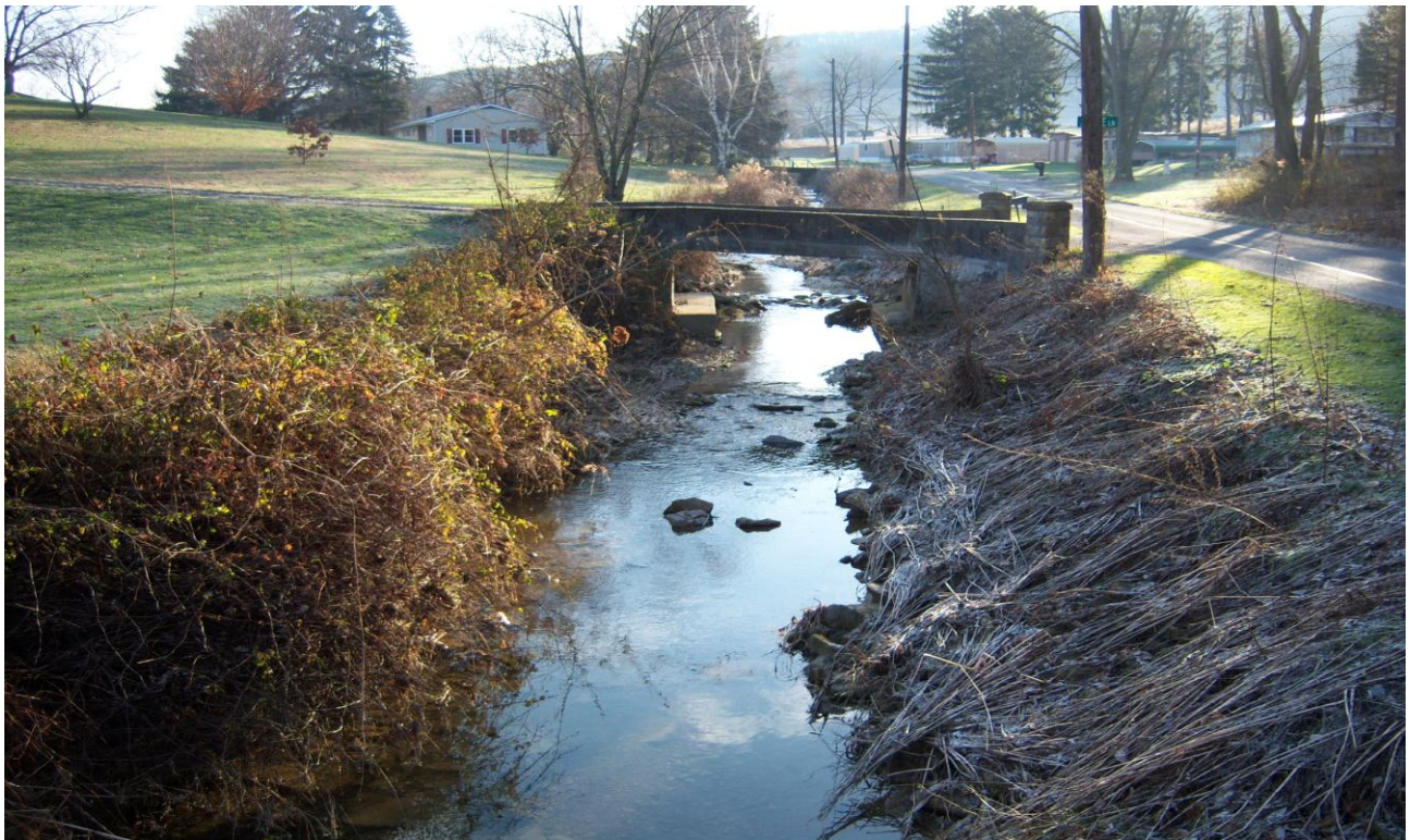
Figure 7. – Mowing up to and deterioration of banks near bridges, culverts, ect.
