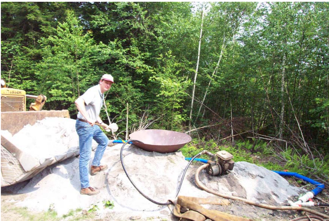
Figure 12. Photograph of limestone alkaline injection into the abandoned Rattler underground mine to pretreat the mine water prior to passive treatment.
