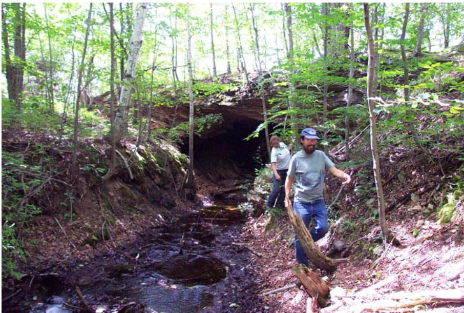
Figure 10. The Anna S No. 1 Discharge of the Anna S Mine Complex, Morris Township, Tioga County.
