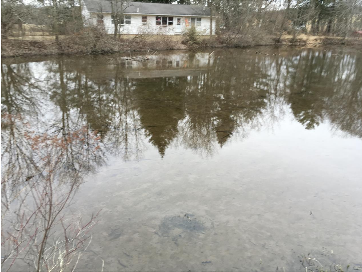
Figure 14. Example of a dammed stream segment in the lower Pohopoco Creek Subwatershed. The ponded area was so full of fine sediment that it nearly reached the top of the dam, so it was assumed that this pond no longer functioned to accumulate sediment. Stream substrates above and below the ponded area appeared to be rocky and free of major fine sediment deposition.
