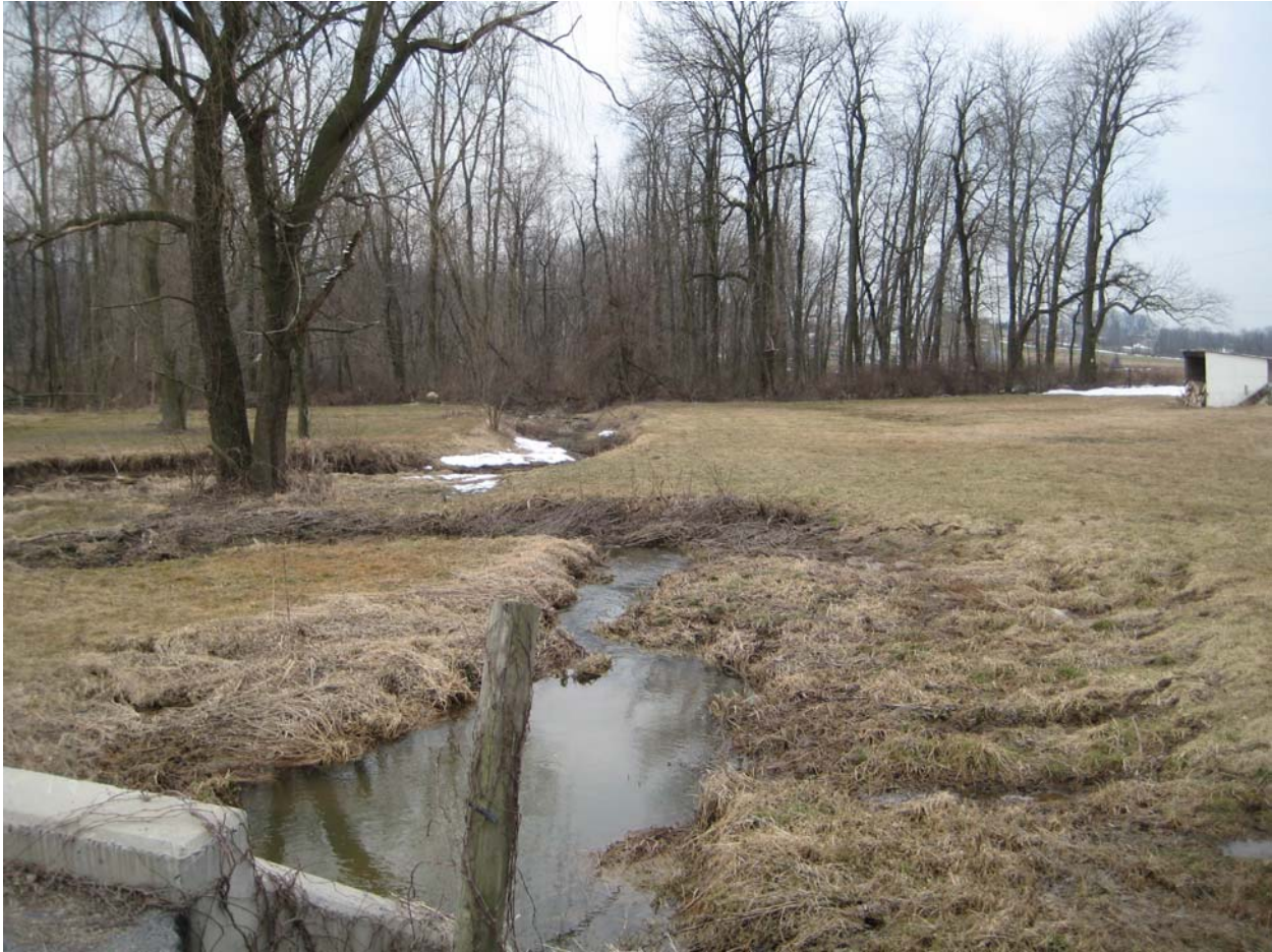
Figure 4. Evidence of Lack of Riparian Vegetation and Streambank Erosion in the Little Swatara Creek Watershed
