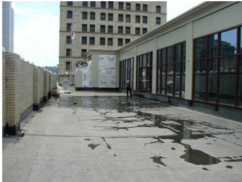
Figure 6.11-3. Ponding of water on a standard rooftop
